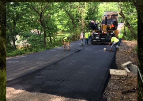
Pavement repairs along transmission line route on McKibbin Street on east end of project.
