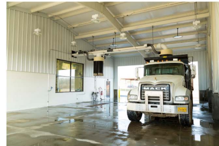
The 8,000 square foot solids handling building includes an operations floor, chemical storage area, office space, electrical room, and a drive through solids loading bay.
