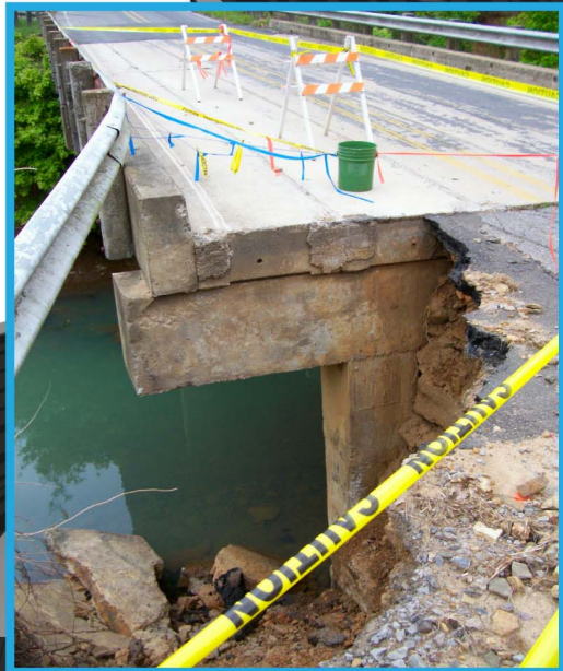
Rock Creek Bridge damage near Mulberry, AR
