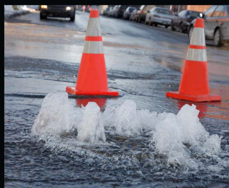
Surcharging can result in sanitary sewer overflows
