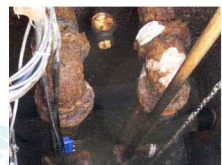
The ductile iron pipe was failing due to corrosion caused by sulfuric acid.
